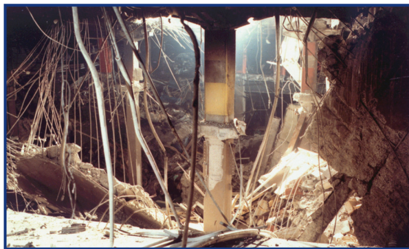
The resilience of a column in the aftermath of the 1993 World Trade Center attack.
